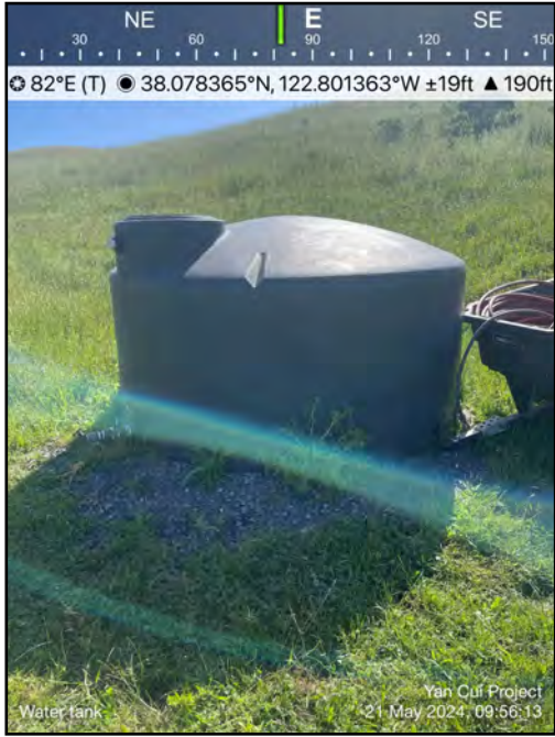
Photo ID: 7 Photo Description: Water tank
