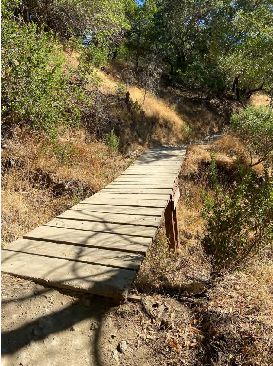
Photo 5: Existing Broken Dam Trail Boardwalk (to be Removed)
