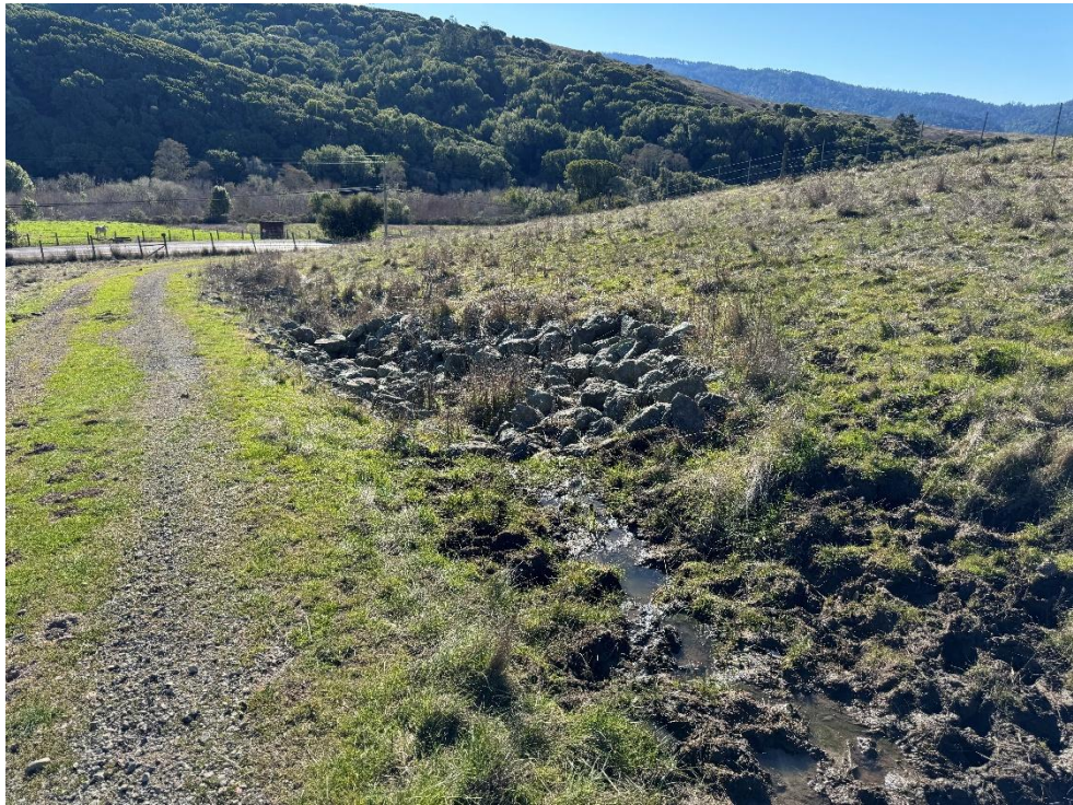
Site Photograph 14 – Looking at pooled water towards culvert adjacent to access easement
