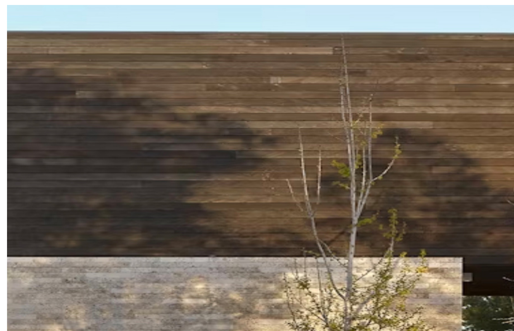
Cedar Wood Siding - Oriented horizontally, dark opaque stain finish (DenseGlass panels installed behind all wood siding).
