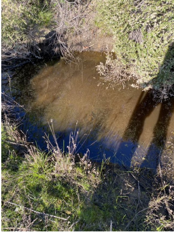
Photograph 8: Standing water in constructed diversion ditch parallel to the eastern slope (drainage segment 1-3). Facing northeast.
