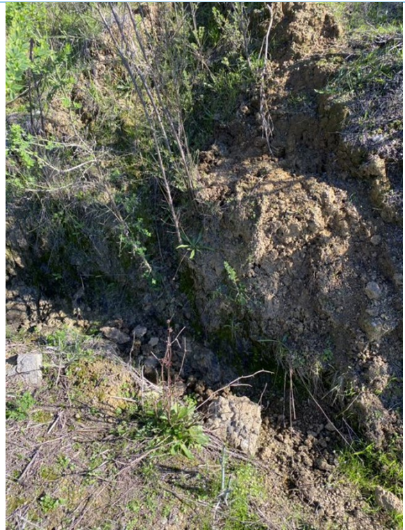
Photograph 7: Scour in Drainage Segment 1-4.
