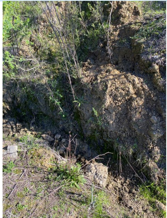
Photograph 7: Scour in Drainage Segment 1-4.
