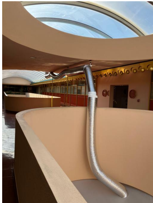
Figure 06: A 2026 leak in an asbestos-containing planter lining on the first floor required enclosing the entire area and managing air flow during remediation.
