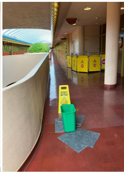
Figure 04. Bucket to catch leaking water during 2026 winter storm.
