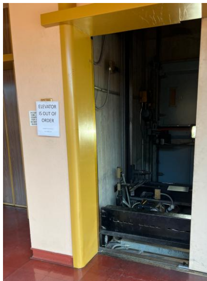
Figure 03. Elevator out of service for 3–4 days in February 2026.
