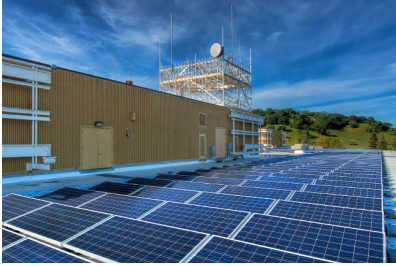
Solar panels installed on rooftop as part of environmental planning project.
