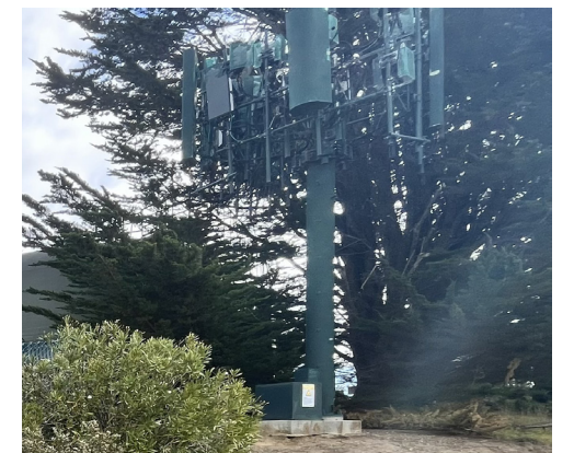
Existing ATS Transmission Tower
