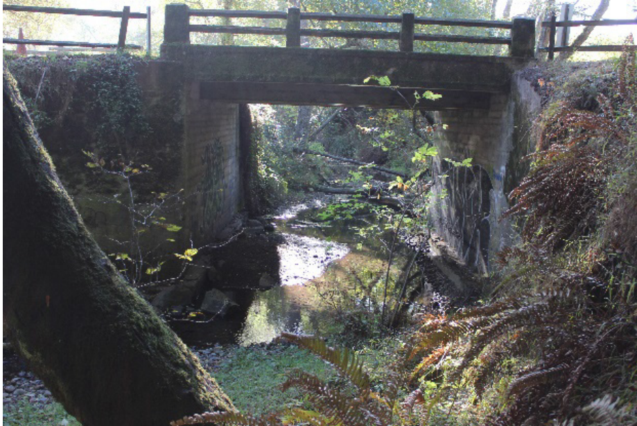
Photo 5. Substandard Redwood Creek Bridge
