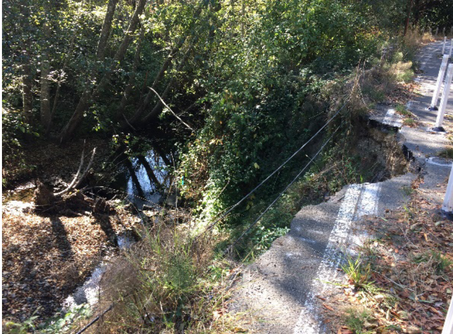
Photo 3. Lane Closure due to Slope Failure
