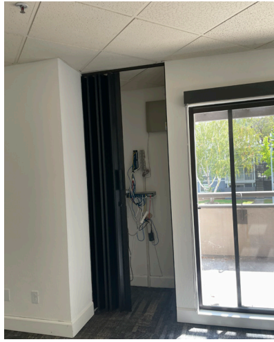
Existing Ad-Hoc Server Closet
