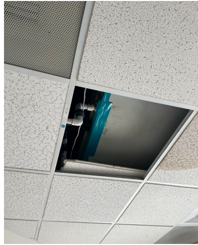
Existing Leaks in Ceiling Damaging ACT
