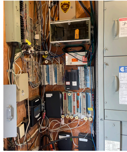
Existing Electrical and Telecom Closet Interior
