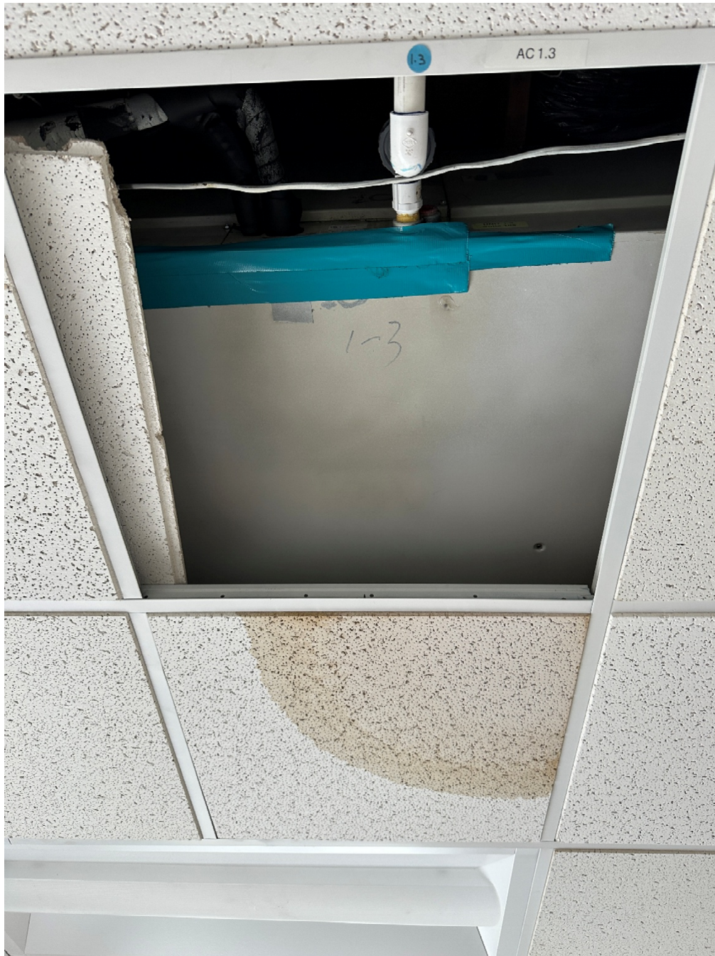
Photo 5: Water Damage at Ceiling with Mechanical Unit Above (First Floor)
