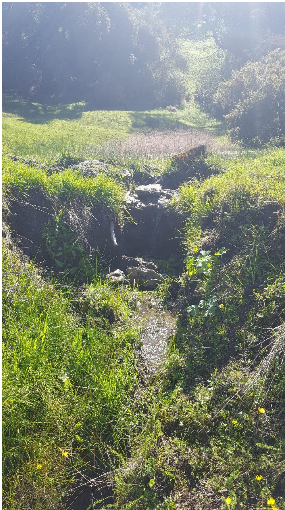
Photo 3. Berm requiring repair at Dry Lake Pond. March 29, 2019.
