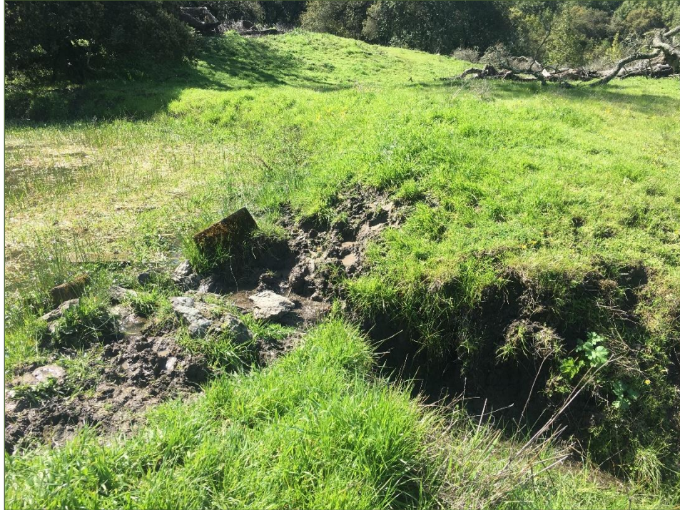
Berm requiring repair at Dry Lake Pond, viewing downhill from top of berm. Note significant downcutting and erosion below berm.
