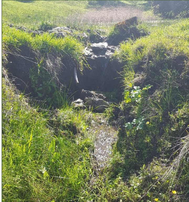
The earthen dam at the outlet of the pond showing signs of erosion.
